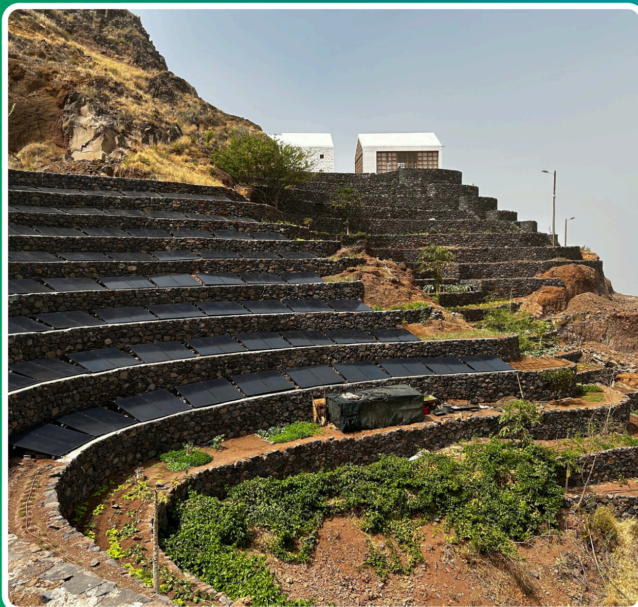
PAINÉIS DO SISTEMA SOLAR FV INSTALADOS THE SOLAR PV SYSTEM PANELS INSTALLED
