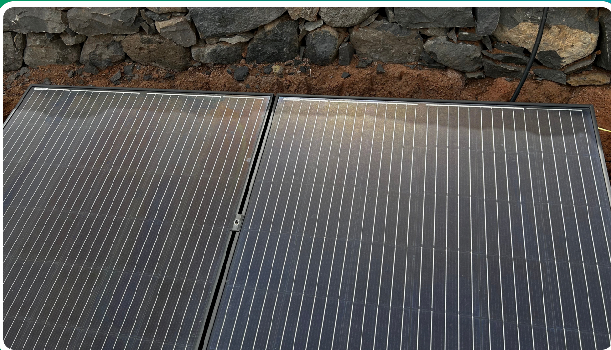
PAINÉIS DO SISTEMA SOLAR FV INSTALADOS THE SOLAR PV SYSTEM PANELS INSTALLED
