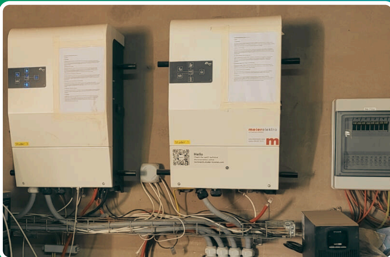
EQUIPAMENTOS DO SISTEMA FV INSTALADO INSTALLED PV SYSTEM EQUIPMENT
