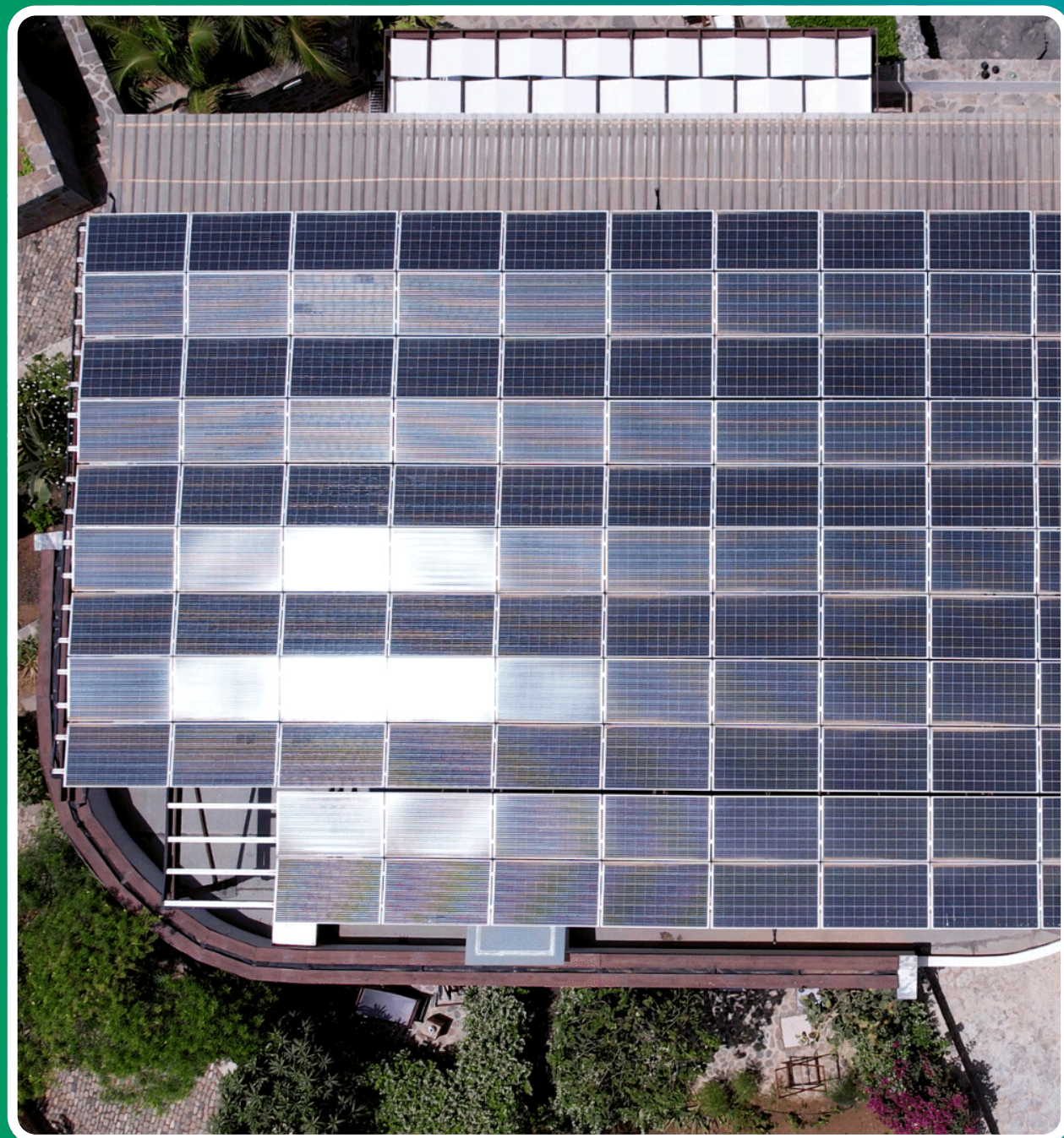
VISTA AÉREA DO SISTEMA SOLAR FV INSTALADO AERIAL VIEW OF THE INSTALLED SOLAR PV SYSTEM
